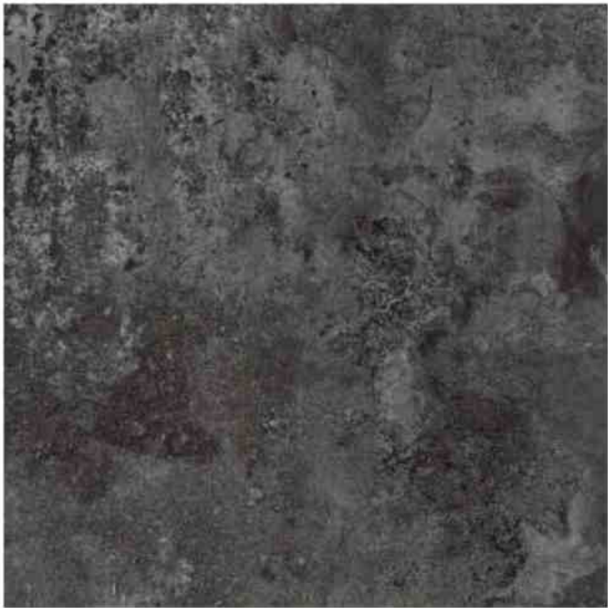
9704 - MG | Weathered Rust
